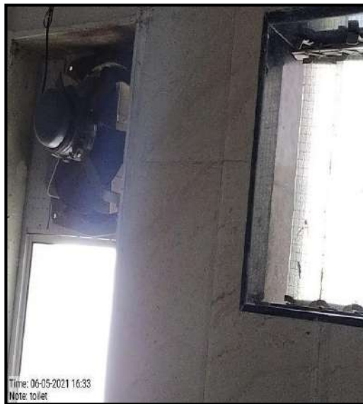
Ventilation in toilets
