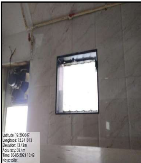
Ventilation in toilets
